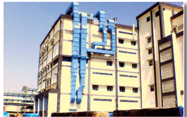
Indorama Chemical Complex at Nagpur. Hot and cold insulation and complete HVAC ducting system.
