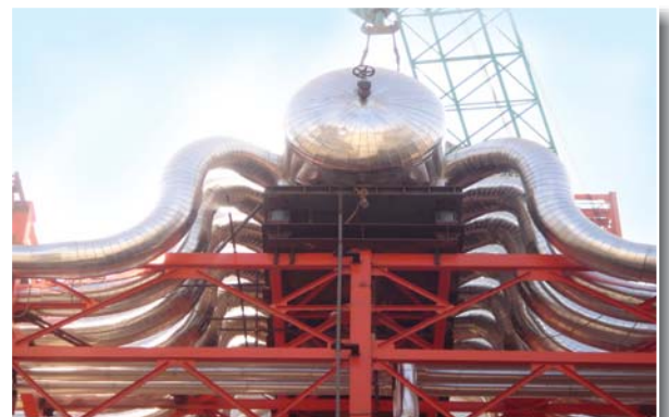
Essar Refinery Project at Jamnagar ISBL & OSBL Project work at Jamnagar Export Refinery.
