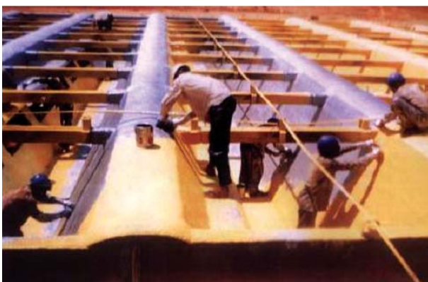
Spray PU & roof insulation & EMA W/P system at ITC Sunrise Bangalore A/c.Larsen & Toubro
