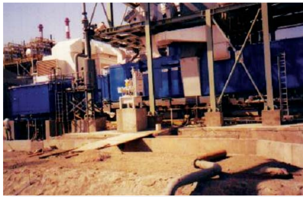
GT Acoustic Enclosure for Reliance Petroleum, Jamnagar.
