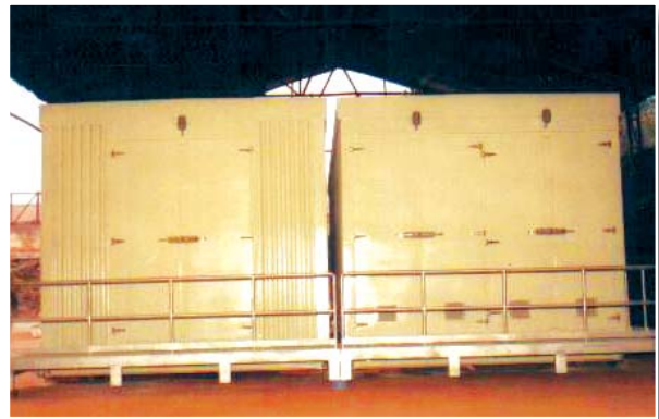
Control Cabinet for PDO Oman GT.
