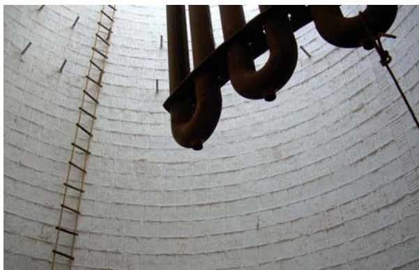
Supercera Ceramic Fibre Module lining for NSU Reboiler Heater at HPCL, Mumbai Refinery
